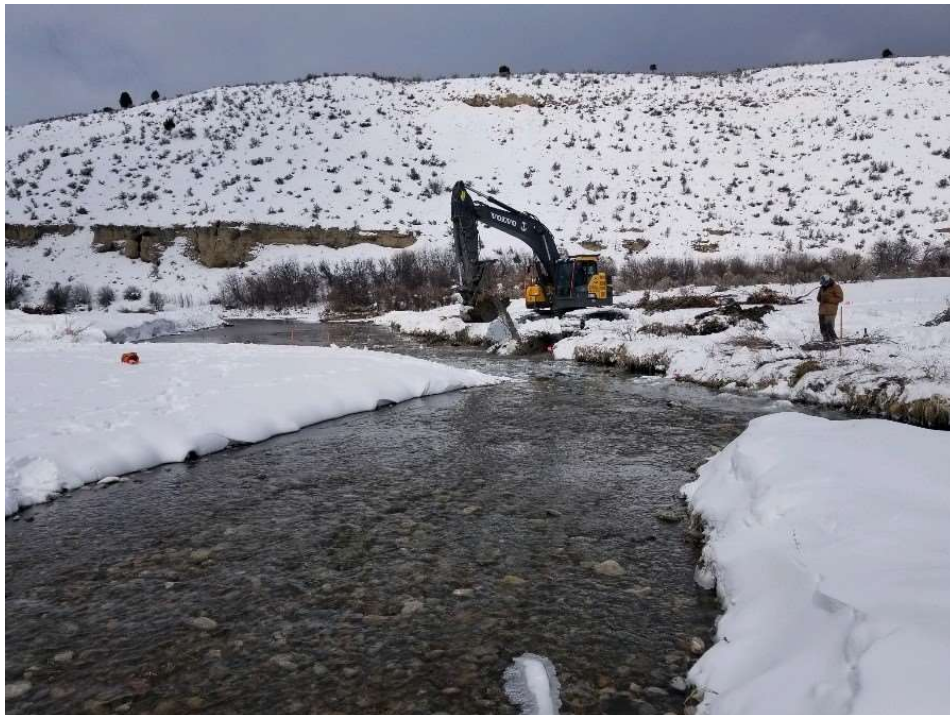
Photo 2. Phase 2, during implementation. Rockin T construction installing large wood and modifying channel.
