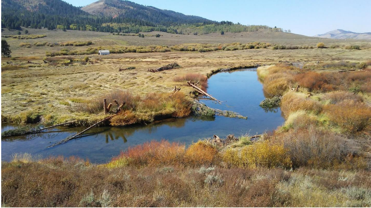
Figure 8. Constructed riffle in the upper right area of the image and whole tree wood treatments in the middle of the image.
