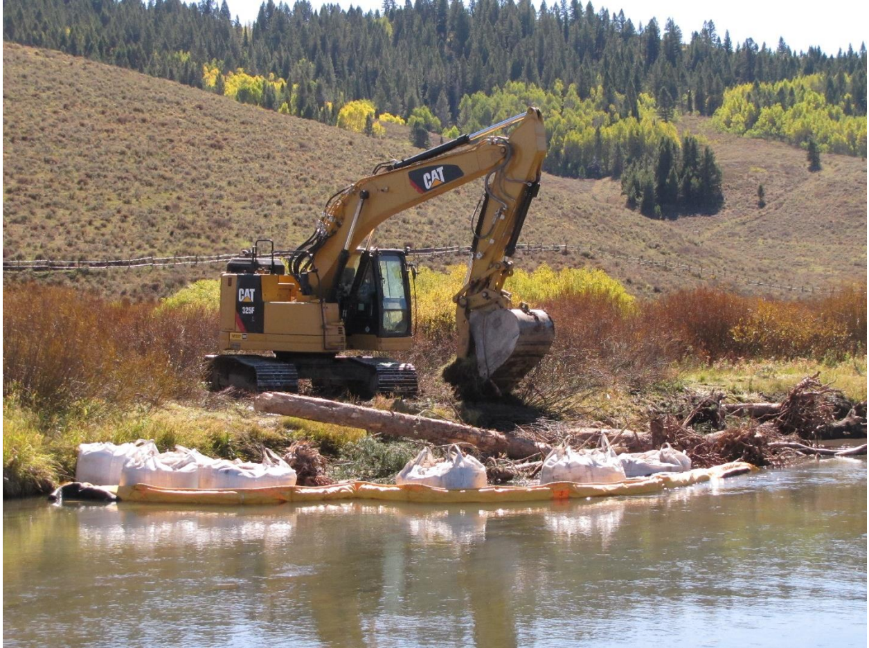
Figure 6. Excavator constructing bank roughening treatment that provides cover for all life stages of Yellowstone Cutthroat and increases bank stability.
