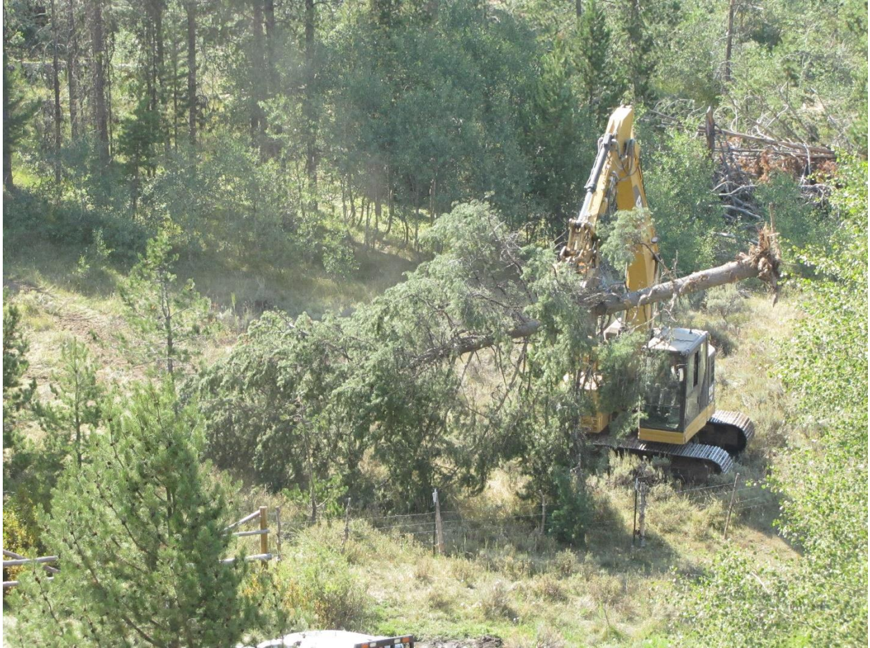
Figure 7. Excavator harvesting whole tree with rootwad from the Blackfoot River Wildlife Management Area.
