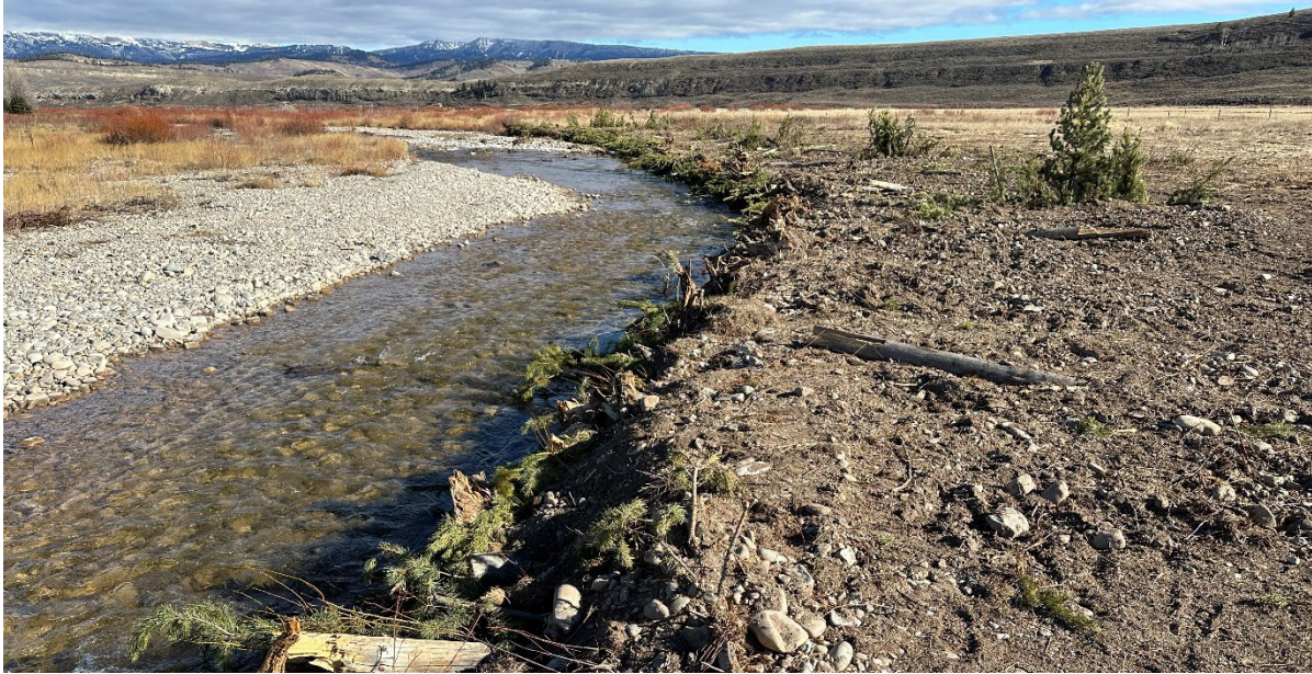
Photo 3. A representative example of a completed brush bank structure with floodplain roughness treatment. In total, 4,247 linear feet of brush bank were installed in 2023 (140 feet remain for 2024).
