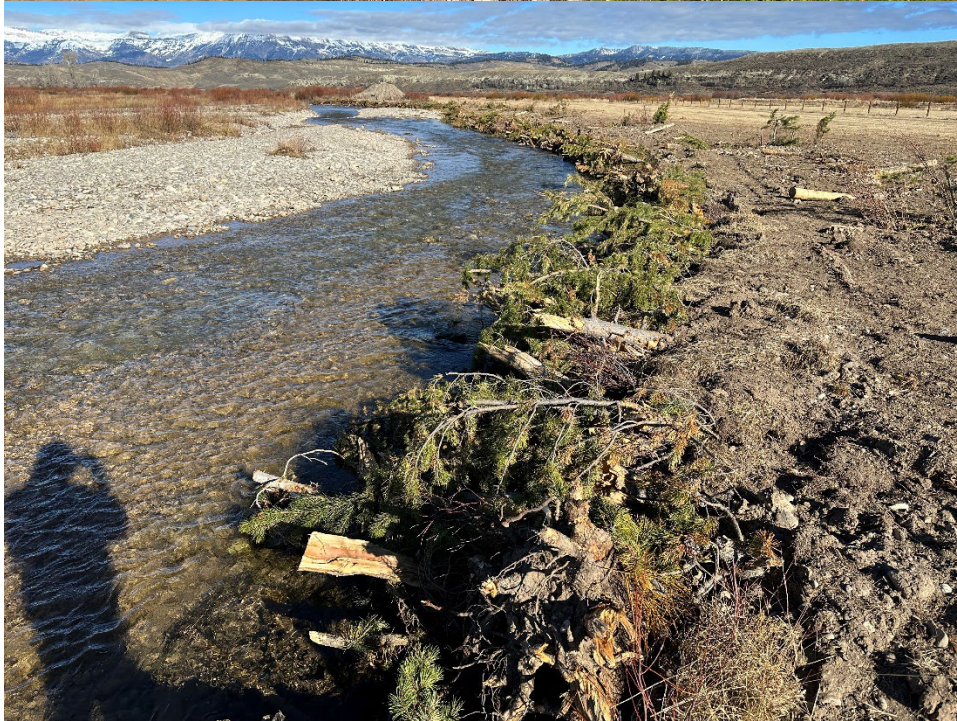
Photo Set 8. Eroding bank along pasture with little vegetative protection (above); brush bank structure (below). Brush banks along outside bends are expected to create good undercut bank habitat for trout.
