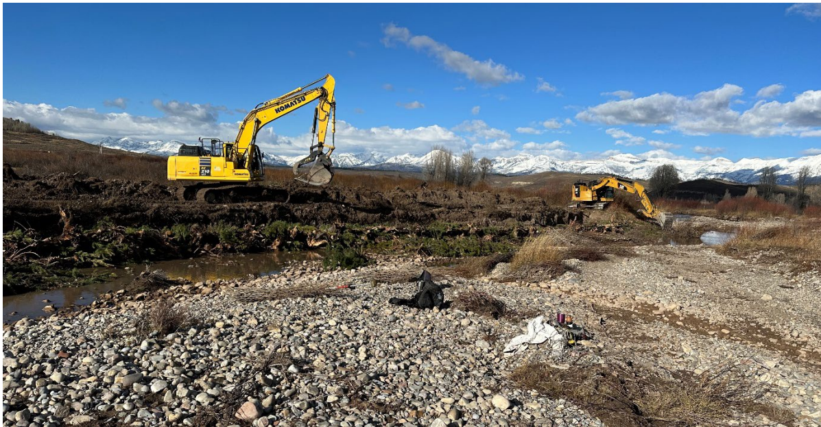
Photo 4. Excavators work to place logs with rootwads into a brush bank structure.
