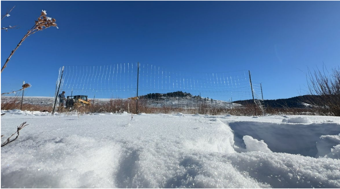
Photo 6. Floodplain revegetation fencing units being completed in December 2023. Fencing units were sited around existing cottonwoods and willows. Once protected from grazing and browsing, they are expected to mature and root, and provide stability and habitat complexity. A total of 26 units were fully installed in 2023, with an additional 41 planned to be completed next year.
