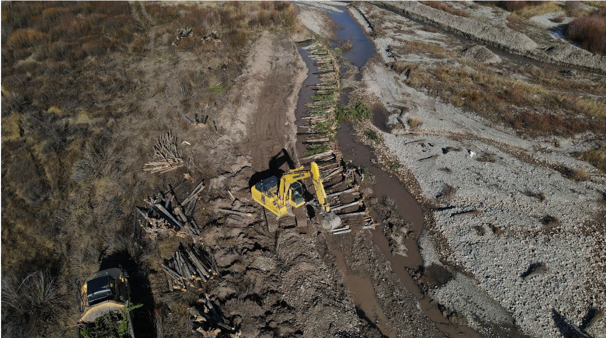
Photo 2. Bioengineered brush bank structures using a combination of medium logs with rootwads, small logs, brush, and willows were installed from October-November 2023.
