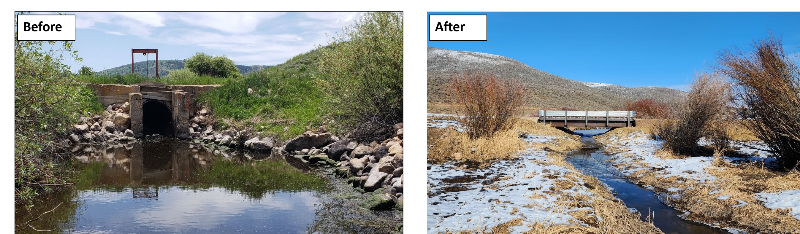
Figure 3. Before- and after- photos of the Stauffer Creek Diversion Dam project (photo credit: Corey Lyman). An earthen dam with a road across it was used to back up water to irrigate over a mile of meadow. A bridge was installed in 2022 to replace the road crossing and irrigation pivots were installed on a hillside to replace the irrigated acreage in the meadow. This project reconnected over 19 miles upstream and will restore a total of about two miles of stream above and below the former dam.
