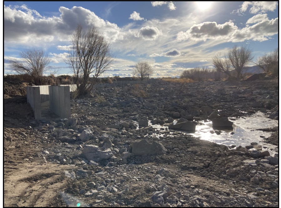
Photo Point: After #2 File Name: 2 Post Project East Channel Below Diversion .jpg Photo Description: East channel looking upstream below the diversion facing south/southwest Photo Date: 12/15/2020
