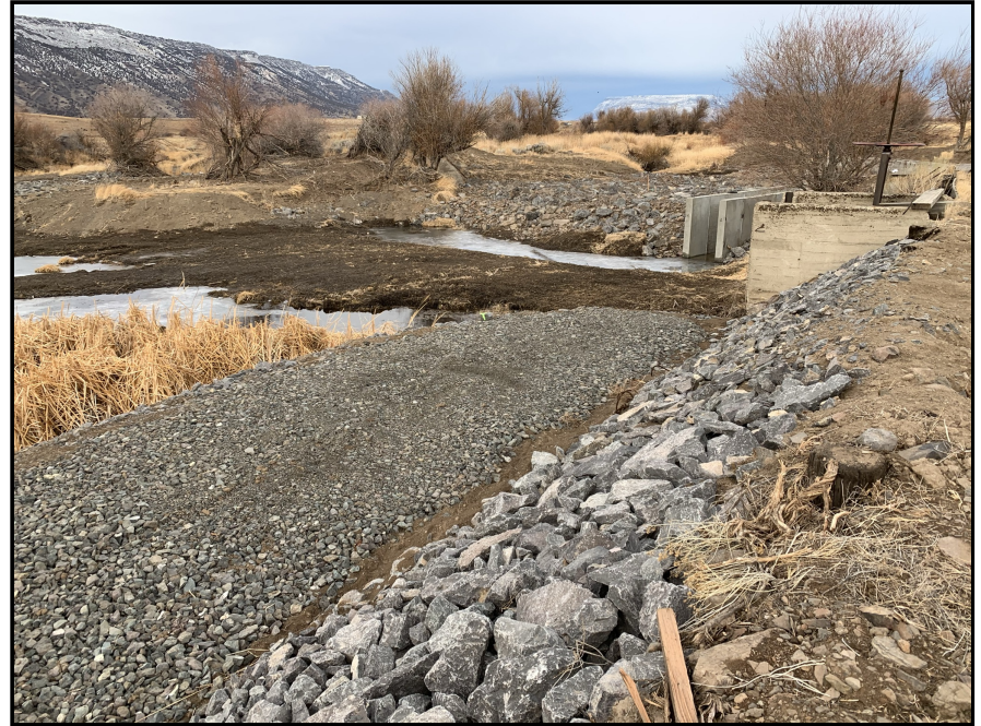
Photo Point: After #3 File Name: 3 Post Project East Channel Above Diversion .JPEG Photo Description: East channel looking downstream above the diversion facing north/northwest Photo Date: 12/15/2020
