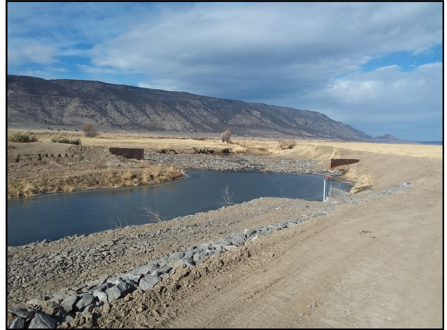
Photo Point: After #2 File Name: 2 Post Project Upstream of Old Weir.jpg Photo Description: Relict Weir upstream of old weir looking north/northwest. Sediment cleanout ramp constructed. Photo Date: 01/21/2021
