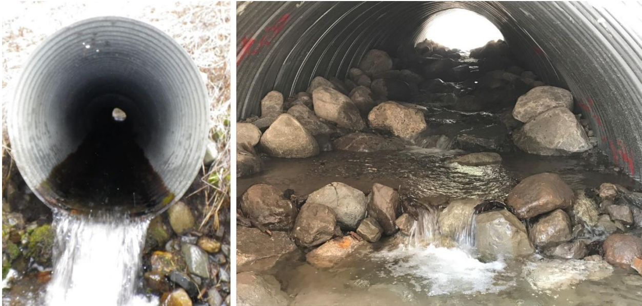
Photo 4. View looking into the Davis Creek culvert prior to (left) and after upgrading to AOP (right). The series of rock weirs and step pools allow fish to pass upstream through this relatively steep culvert.
