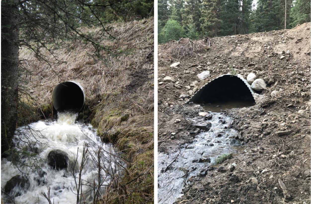
Photo 3. Davis Creek culvert outlet prior to (left) and after upgrading to AOP (right).
