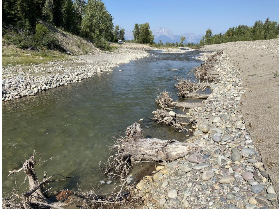
Photo Set 10. Before and after. Steep eroding bank (above), regraded bank with toe rock, logs with rootwads, and willows (below).
