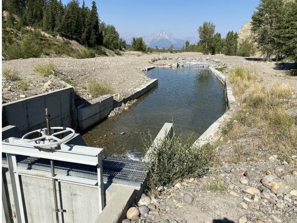
Photo Set II. Previous headgate and sediment basin (above), expanded sediment basin and new fish screen at far end (below).
