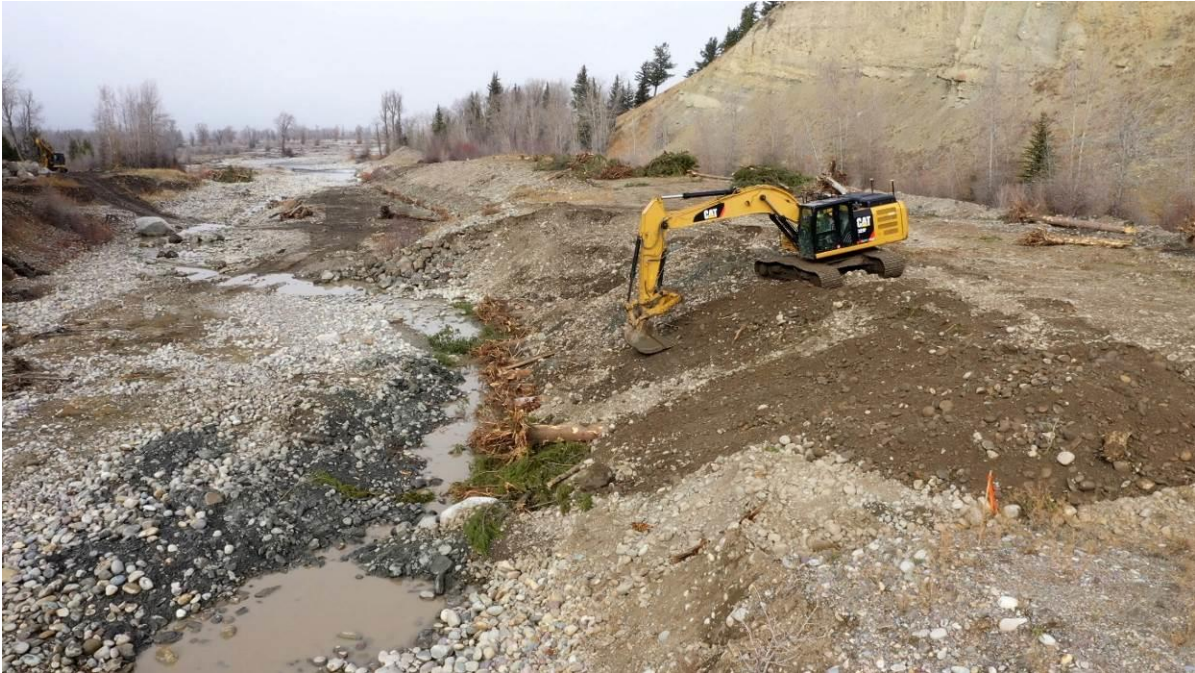
Photo 1. Bank stabilization structures using a combination of wood, rock, resloping, and erosion fabric were installed in November 2021.
