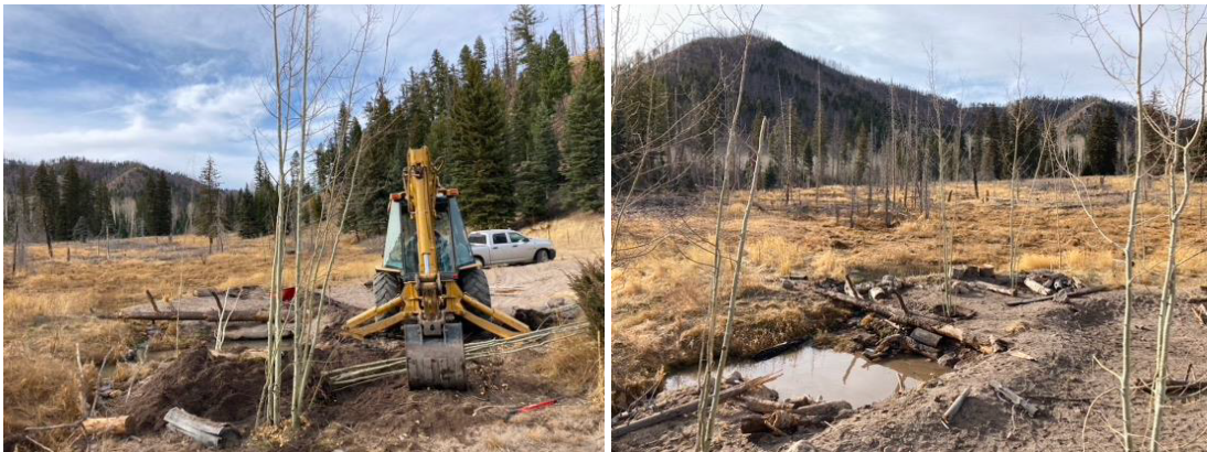
Fig.6) Aspen transplants were placed along newly created ponds to facilitate shade for cover and maintaining cold water temperatures.
