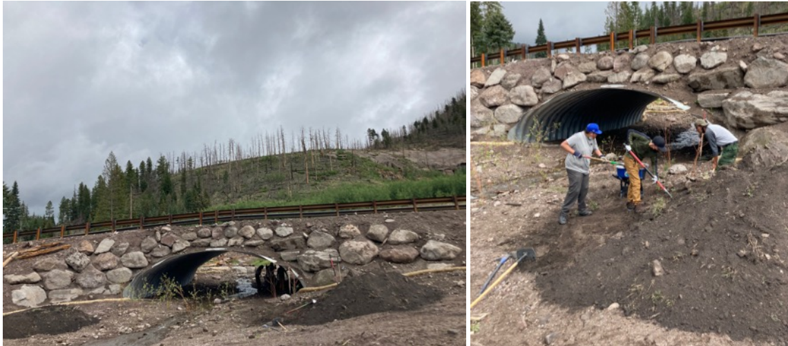
Fig. 2) Field implementation crews began work by developing a bankfull bench and side channel pool to encourage fish passage and facilitate proper stream dynamics under a recently completed bottomless culvert.
