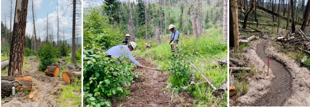
Fig.5) Fish barrier bypass constructed along Turkey Creek. A relic tributary was utilized to direct water around a 6-foot tall debris dam that presented a barrier to fish migration. This bypass channel was created to establish the flow around the barrier to facilitate fish passage. The new channel will be monitored and treated with adaptive management in the future months and years. Adaptive management will prioritize the development of habitat microsites to facilitate fish holding and a bankfull channel with floodplain connectivity to accommodate flow variability.
