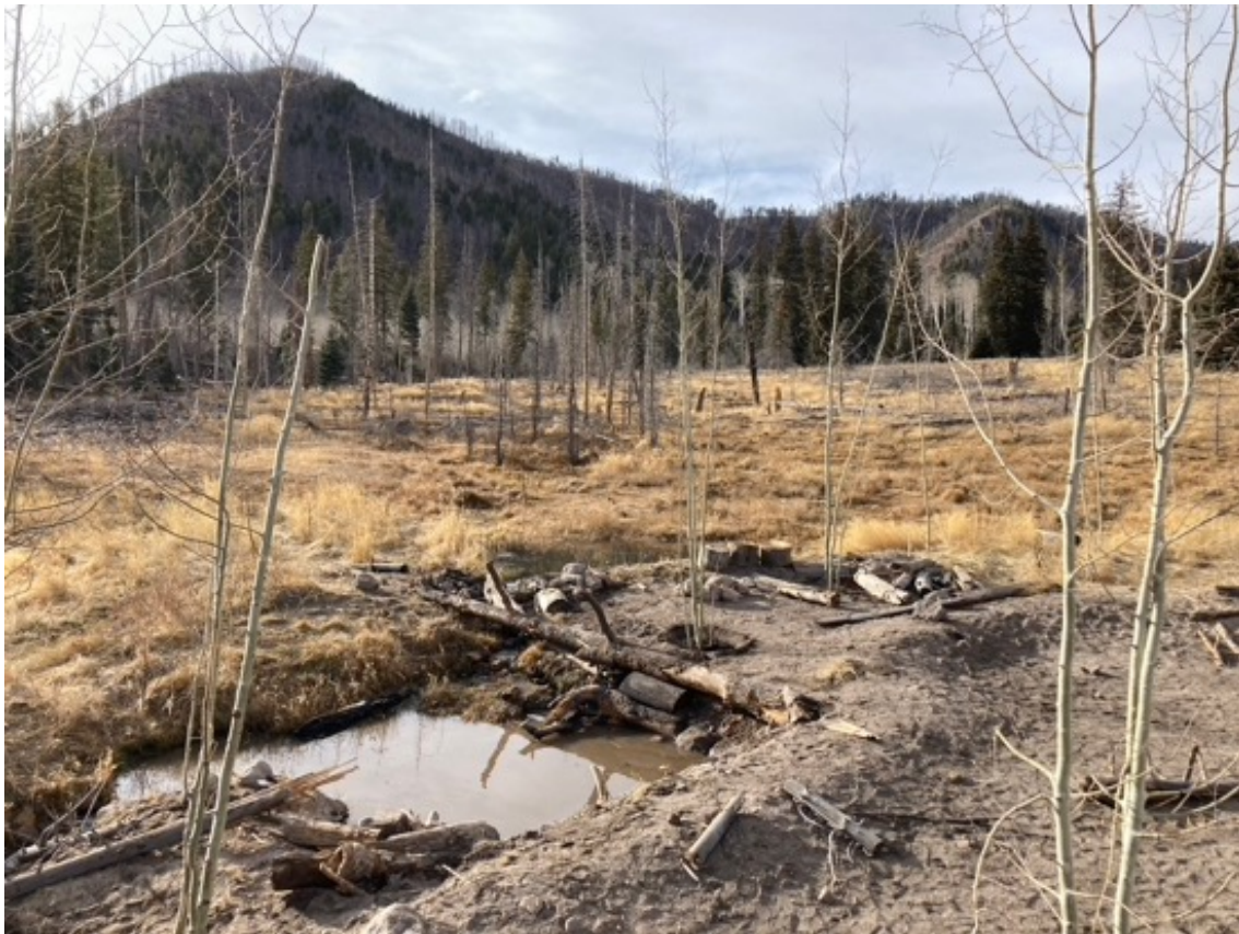
Fig.9) Completed off-channel ponds integrated into relic beaver ponds and wetland complex (December, 2021).
