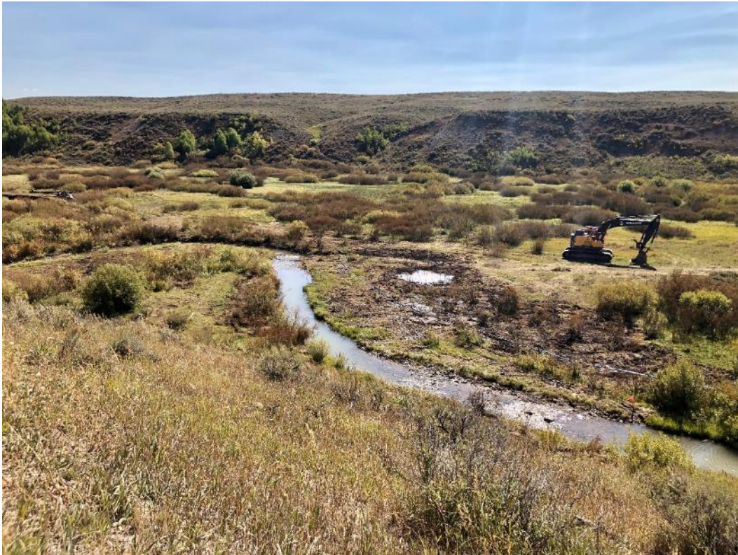
Rockin' T Construction equipment staged to tackle the last stretch of the project in September 2020.
