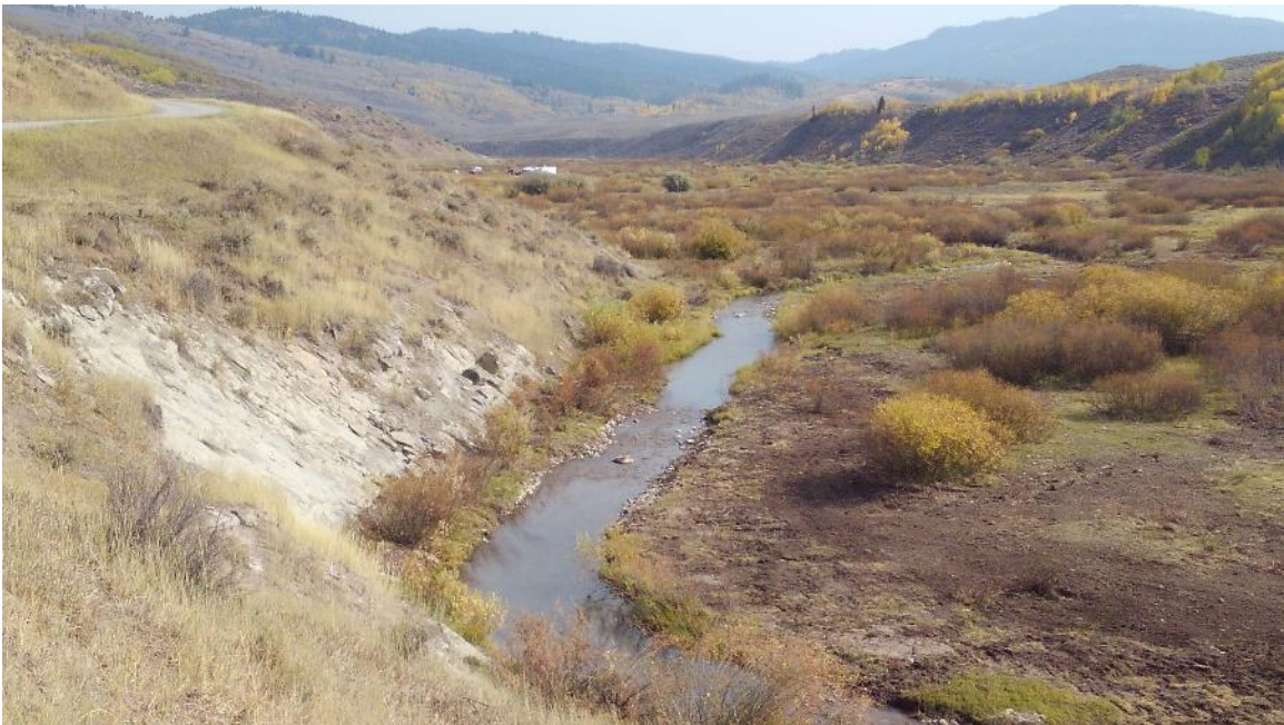
After: A floodplain bench was built to create better habitat, and willows were moved from the inside to the outside bend to protect it from erosive forces and allow for floodplain access on the inner bend.
