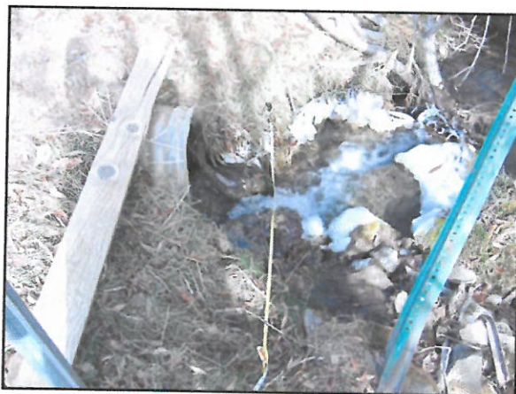
Figure 2. Hutch Creek, pre-project. Culvert is undersized and outlet is poorly sited over rip-rap.
