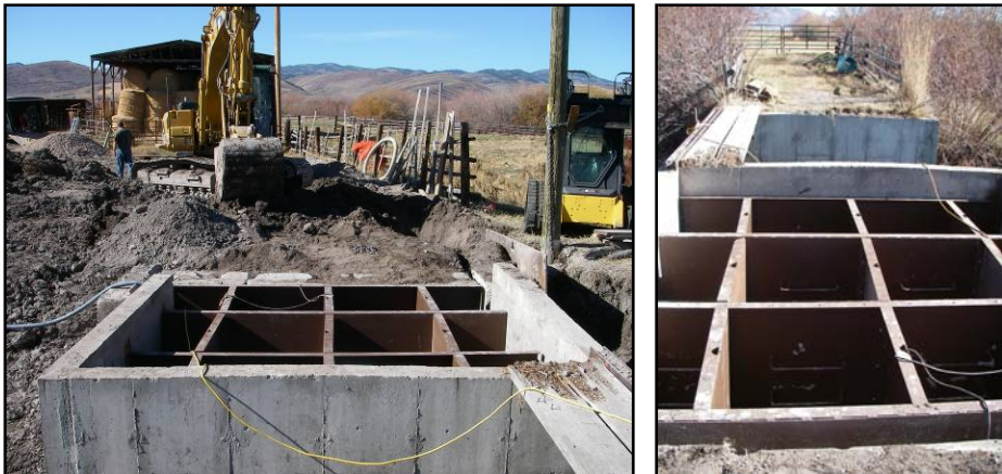
Transtrum Irrigation Diversion during (left) and immediately after (right) installation. This configuration allows for upstream fish passage without significantly increasing the footprint of the existing structure.
