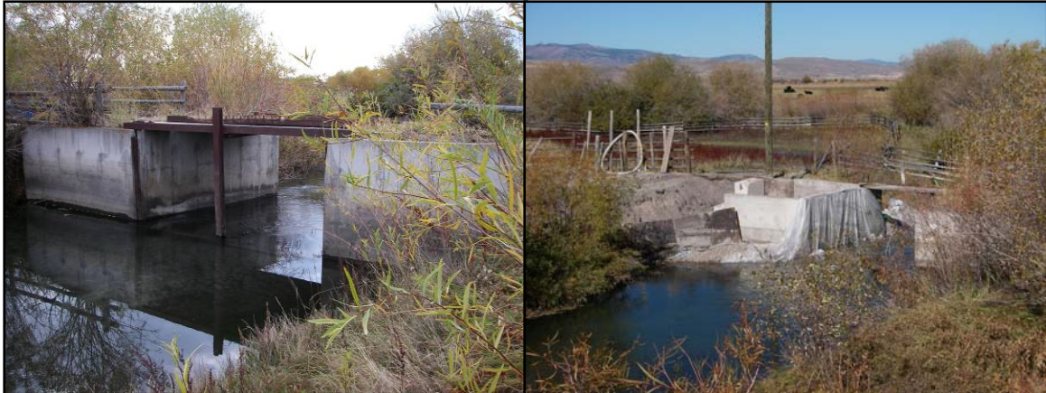
Transtrum Irrigation Diversion before fish passage restoration (left), and during construction of new fish ladder (right).
