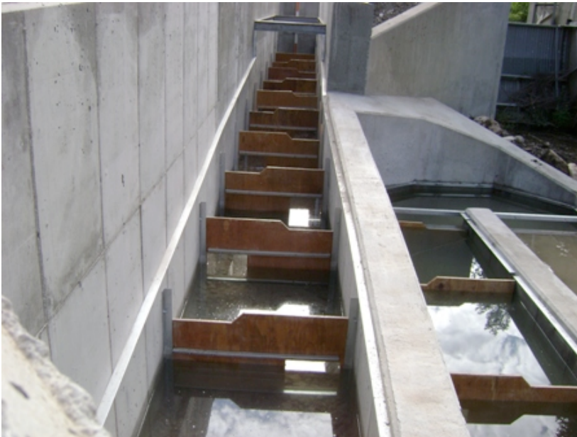
Orifice weirs in fish ladder with partial flow.
