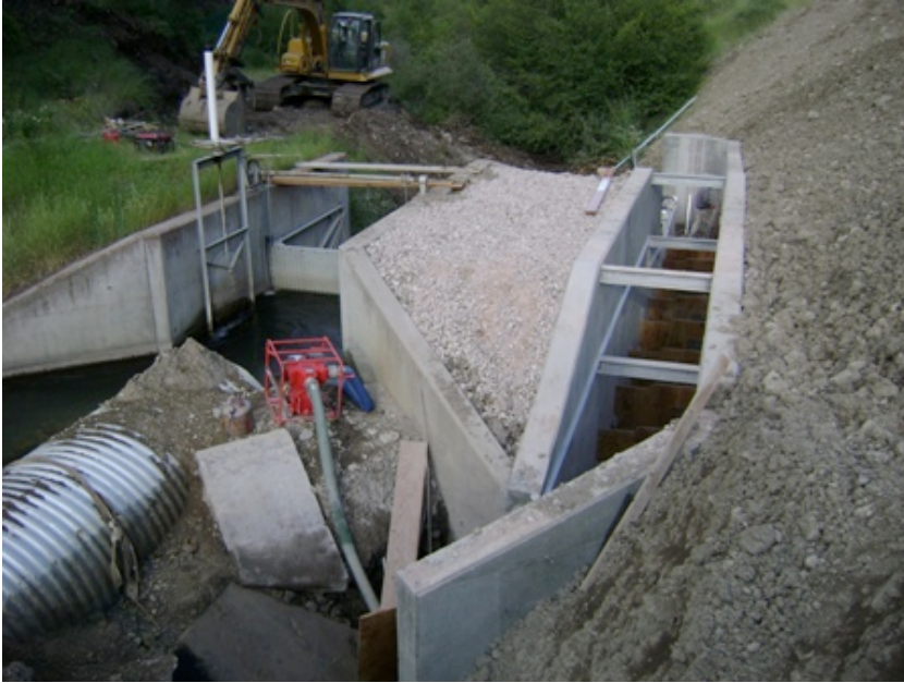
Water diversion into hydroelectric diversion intake so construction crews can work in the dry.
