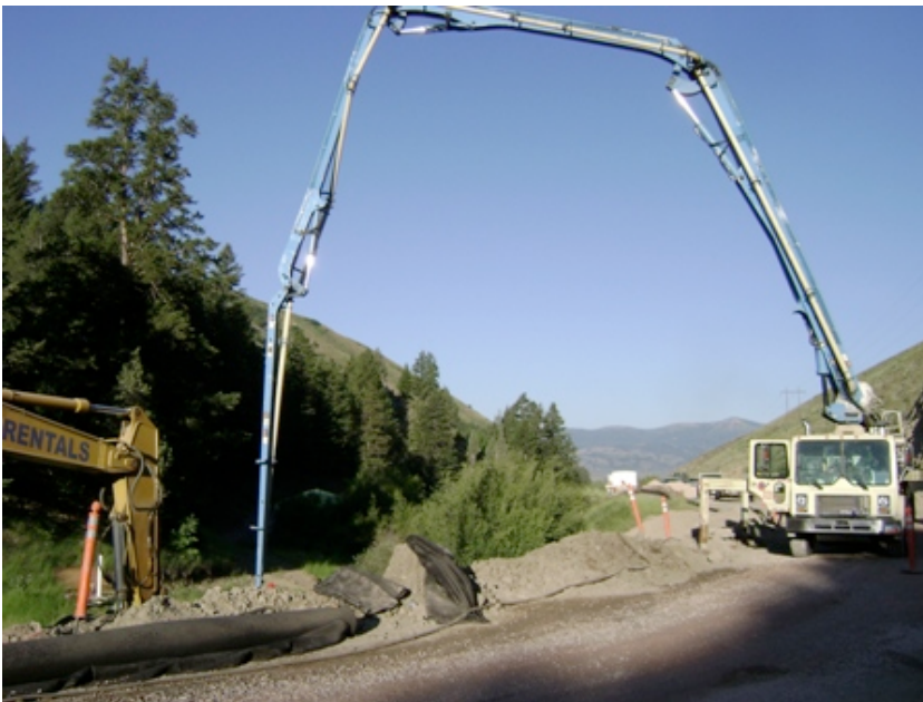
Concrete pumper pouring the floor of the fish ladder facility around the Georgetown hydroelectric diversion headgate, July 2009.
