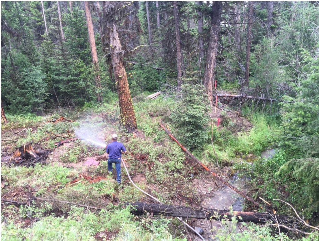
Photos 5-6: Backfill and armoring of the culvert and contractor watering transplants and sod mats to complete finish work on the riparian area.
