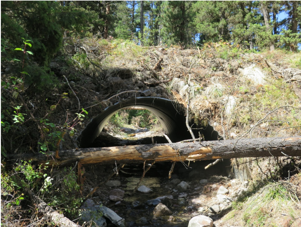
Photos 1-2: Photo point showing existing condition of the culvert outlet compared with upgraded pipe arch. Project was completed in mid-August, 2016.
