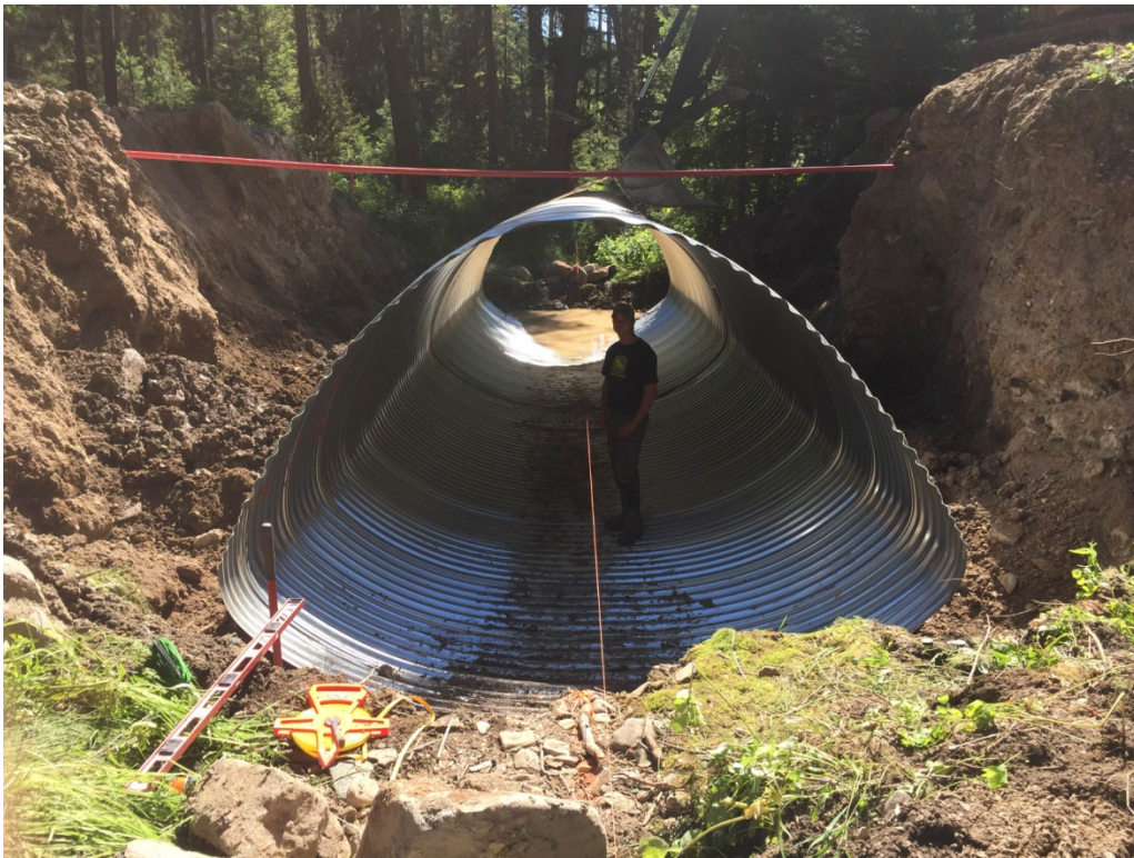
Photos 3-4: Construction progress showing site condition once culvert was removed and the placement of new pipe arch.
