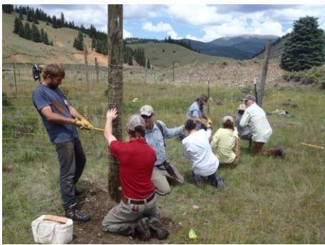
Volunteers work to repair a damaged grazing exclosure, August 2011.
