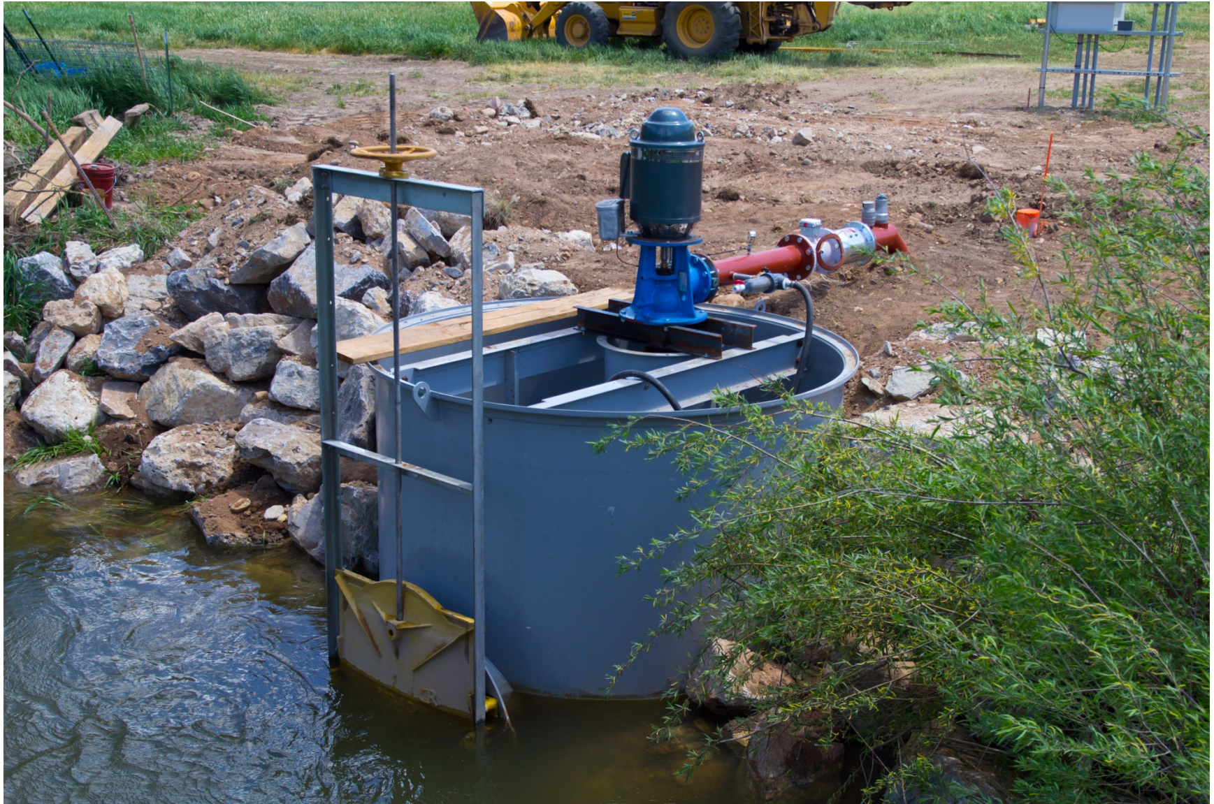
Figure 5: The new screened stream-side pump on the Chalk Creek mainstem.
