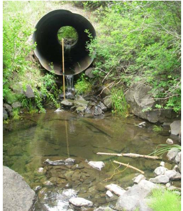
Photo of Perched Culvert before replacement
