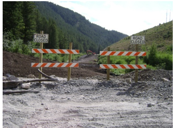
The view from the upstream end of the project site from an untreated segment of the old road.
