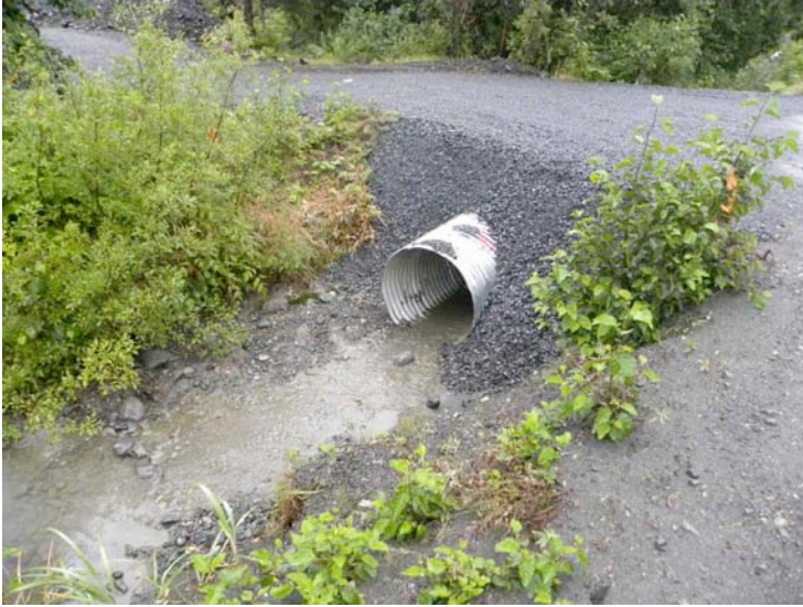
Figure 12: Looking downstream at the upstream side of the Bartley driveway culvert. This ditch now drains stormwater from the City Baler.
