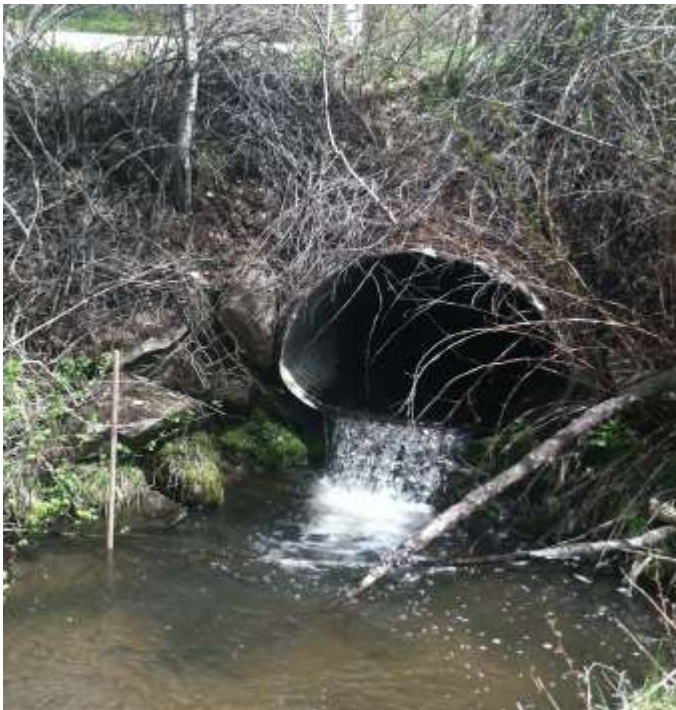
North Fork Dry Cottonwood Road 85 culvert to be replaced with AOP culvert in summer, 2018.
